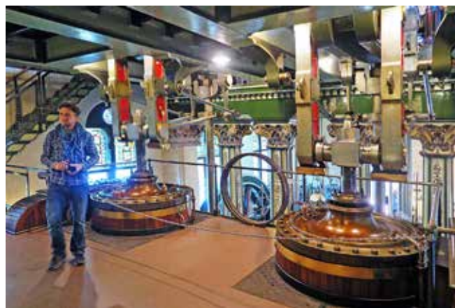
Papplewick: The cylinder floor of the two Boulton and Watt pumping engines. Photo Clive Penfold
